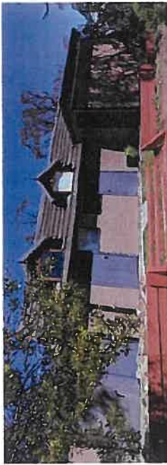
FIGURE 11.1: UNIT 58 - NORTH ELEVATION (GULLY FORM PARTIALLY OBLSCURED). MODIFIED EXTERNAL FINISHES AS SHOWN
