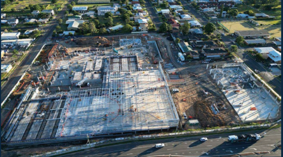
Aerial view from the south. Structural steel to Pour E, Pour G formed and ready for reo, PT and services, Pour K concrete being placed.
